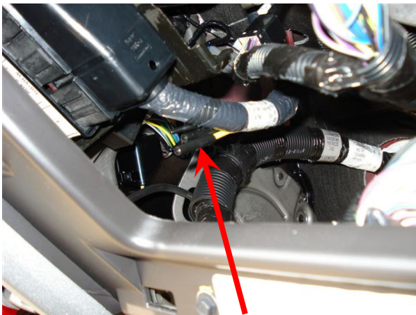
Four Blunt Cut Wires (Figure 1)
